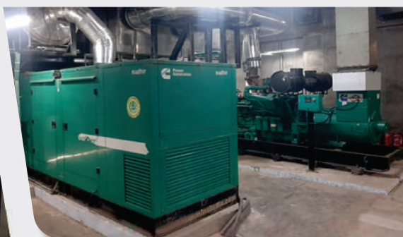
Retrofit Emission Control Devices on all generators to minimize pollution.
